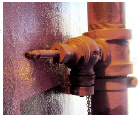
This Class I hose station outlet needs attention to make it usable for the fire service. Photo courtesy of Byron Blake.
